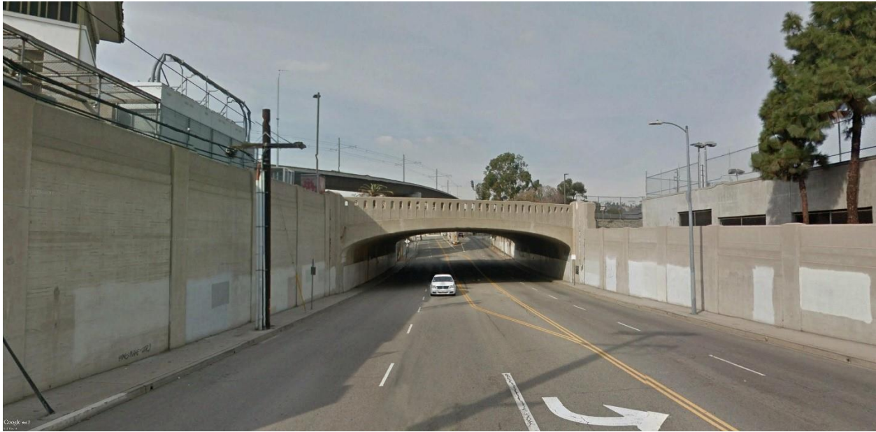
Figure 3.4-26. Key View #2a – Vignes Street Bridge (view looking west toward bridge) Existing Conditions
