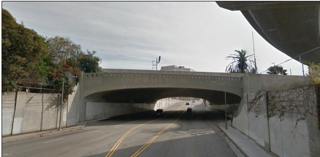
Figure 3.4-29. Key View #2b – Vignes Street Bridge (view looking east toward bridge) Post-Project Conditions with New Bridge
